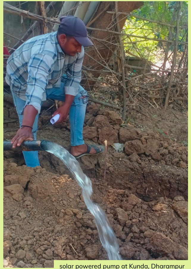
solar powered pump at Kunda, Dharampur
