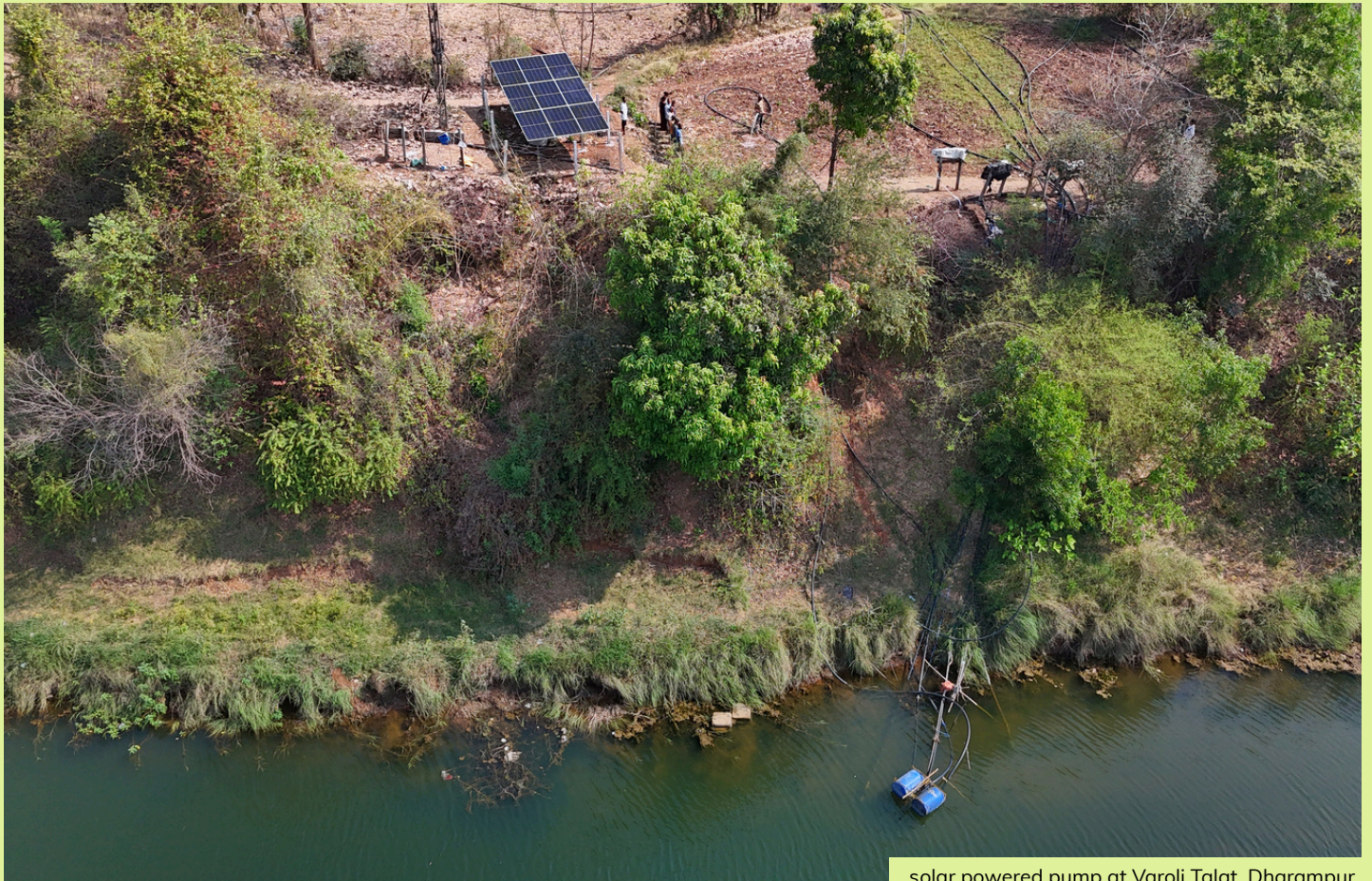
solar powered pump at Varoli Talat, Dharampur
